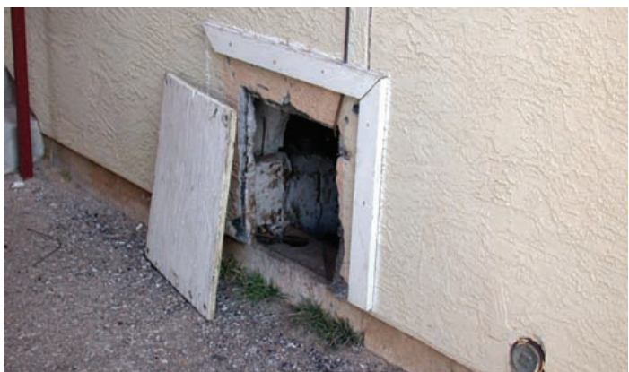
Access panels should not be left open
